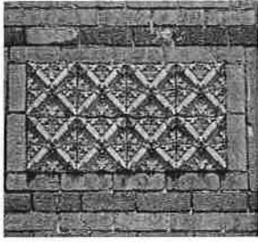
Terra Cotta work embedded in the chimney
